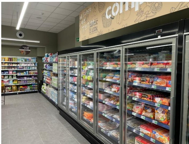
Exkal cabinets (multideck, freezers) and display counters
